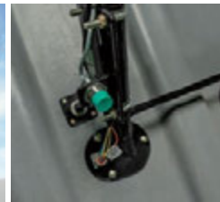
Low level tank sensor.
